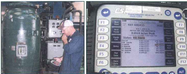
Above: Level 2 Vibration Analyst conducting a vibration survey on a vertical motor in-house for repairs. Above right: CSI 2130 dual channel vibration analyzer:
